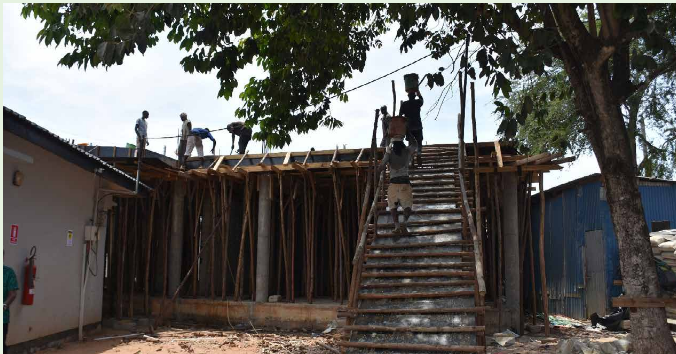
Construction work for new offices of the Media Council of Tanzania in progress
