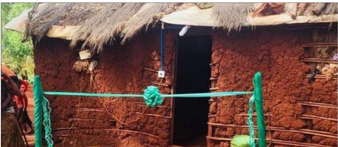
Local houses installed with electricity
